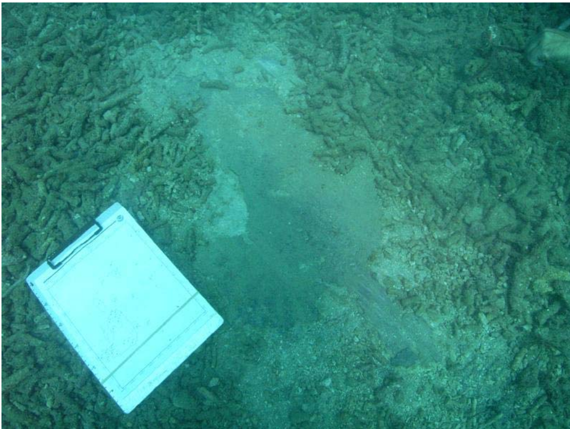
Figure 6. Area of anti-fouling paint that needs to be removed, at letter J in Figure 3.
